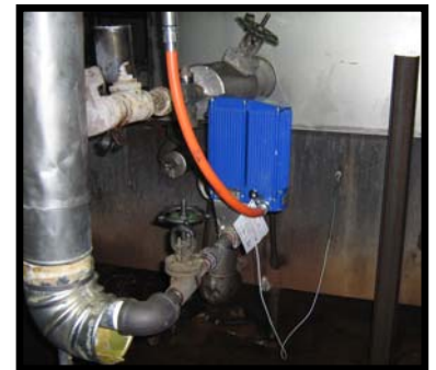
Traditional Thermostatic and Emech Steam control solution
